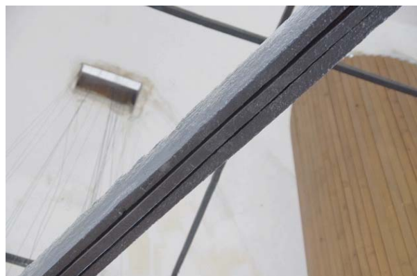
Figure 7: Tie rod showing forging (Lorenz 2012)
